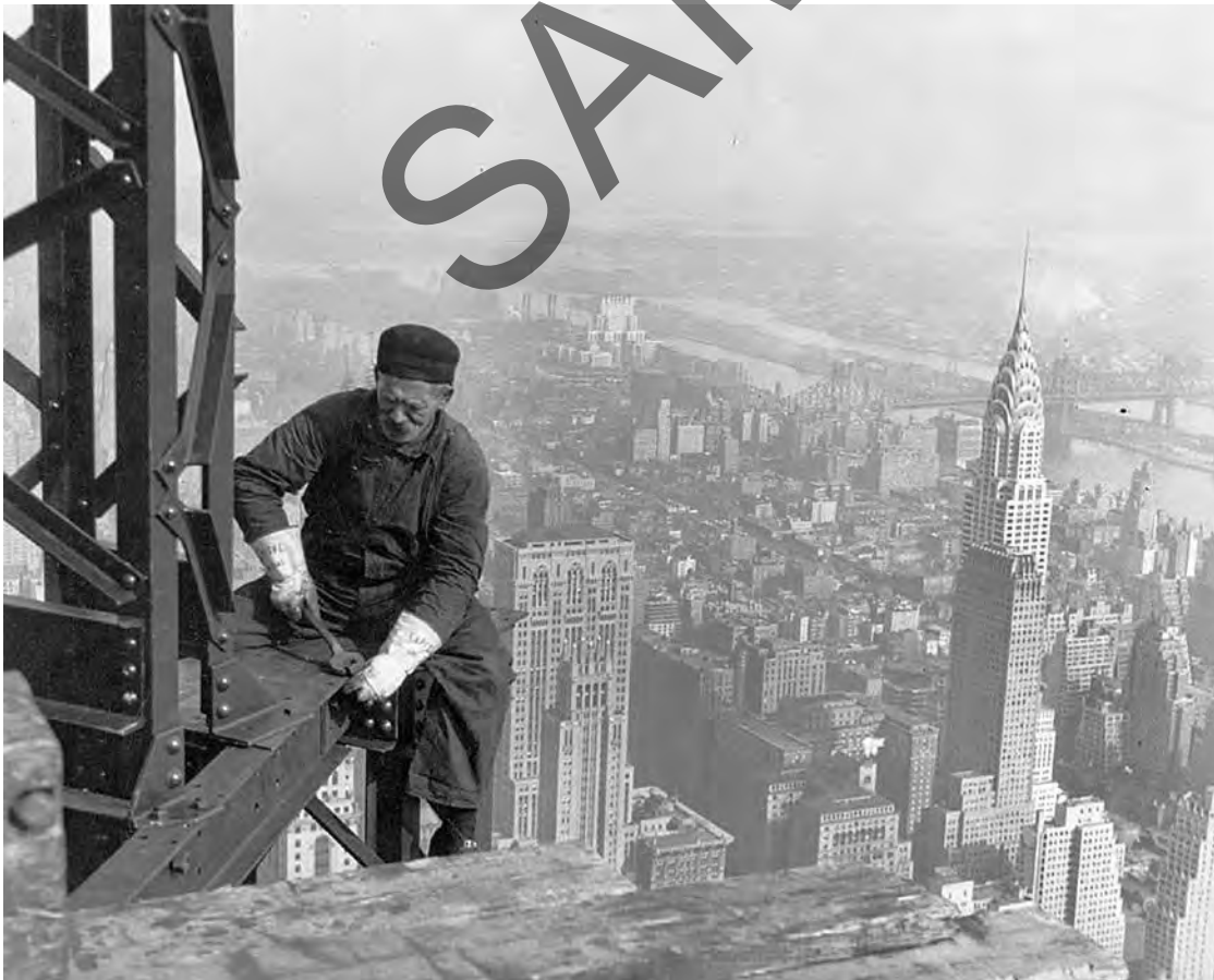
Workman on the Framework of the Empire State Bldg., with the Chrysler Bldg. off to the distance, 1930.
